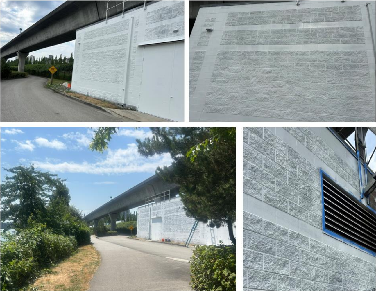
Figure 2: After nano paint application
