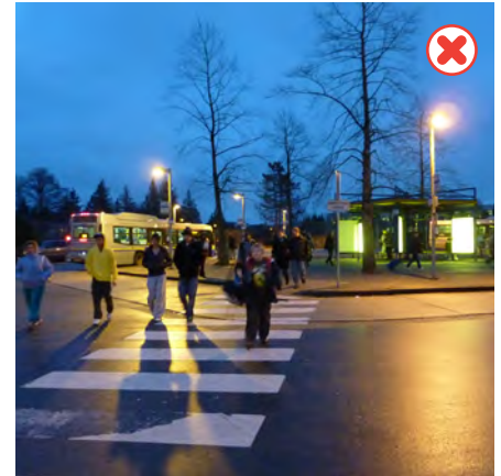
Poor integration with third-party lighting resulting in glare and dark areas. Edmonds Station Bus Exchange, Burnaby.
